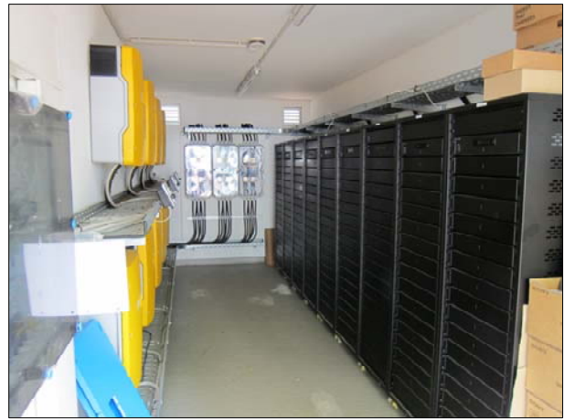
Figure 5: Photograph of the battery racks inside the container (large container version).
