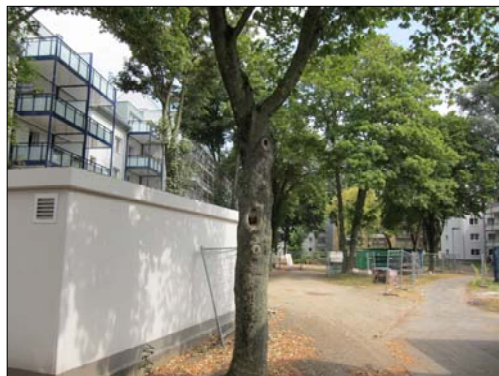
Figure 3: Photograph of the common yard between the houses as well as one of the battery containers.
