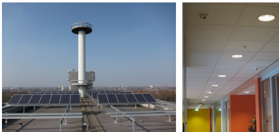
Figure 10 Photos of the demo DC grid installation: Left : Photovoltaic panels. Right : DC driven LED lamps.
