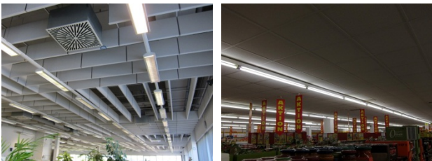
Figure 1 Typical ceiling of an open space office ( left ) and in a supermarket ( right ).
